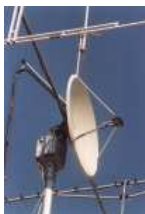
"HAM" radio application with parabolic and yagi antennas
